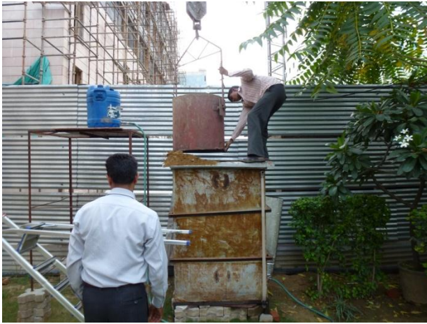
With the help of a crane and some construction workers, sand is poured into the tank.
