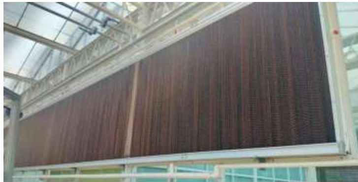
Figure 4 Greenhouse Greenhouse Cooling Water Curtain
